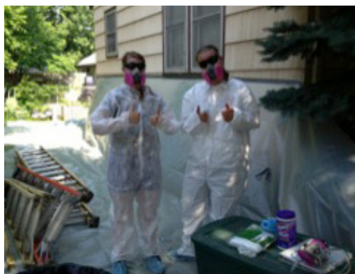
The crew suits up for lead-based paint safety at a Winona-Fillmore Habitat repair project.
